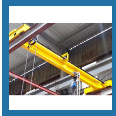
Overhead HOT Cranes
