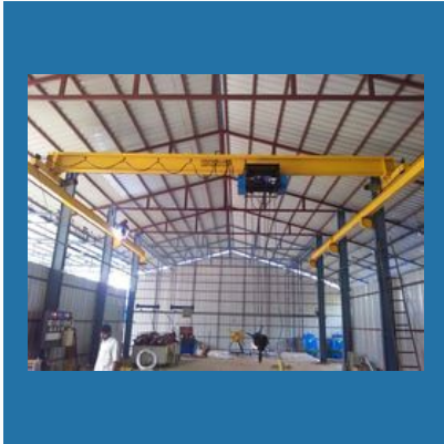
Single Girder EOT Crane
